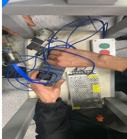
Figure 27: Wiring Correction Source: Own elaboration
